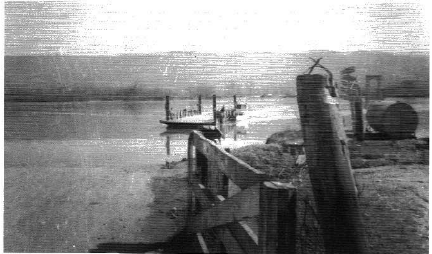
1961, the beginning construction of the Snodgrass Bridge Pier at the Caperton Ferry near Stevenson.
