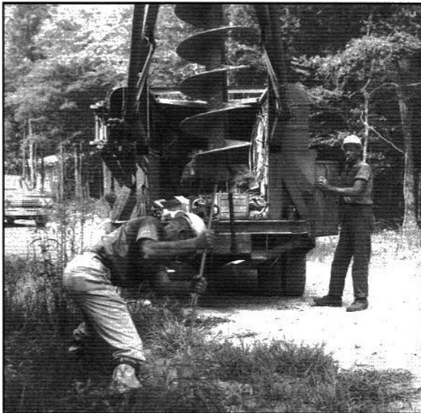
Johney King and Fred Keller (standing next to truck) begin work on setting a power pole in the early 1960's.
